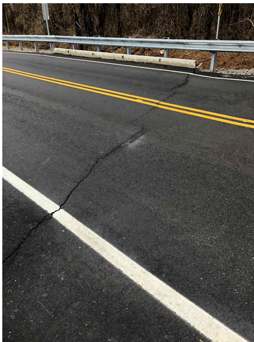
Pavement Cracking at East Abutment Connection
